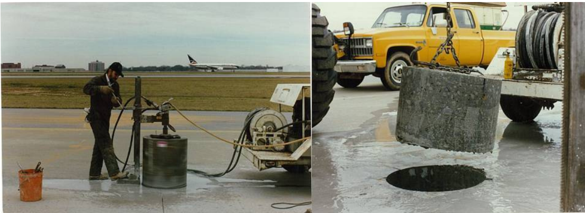
Figure 8 – Large 26-inch Diameter Core for Taxiway Cracking Investigation
