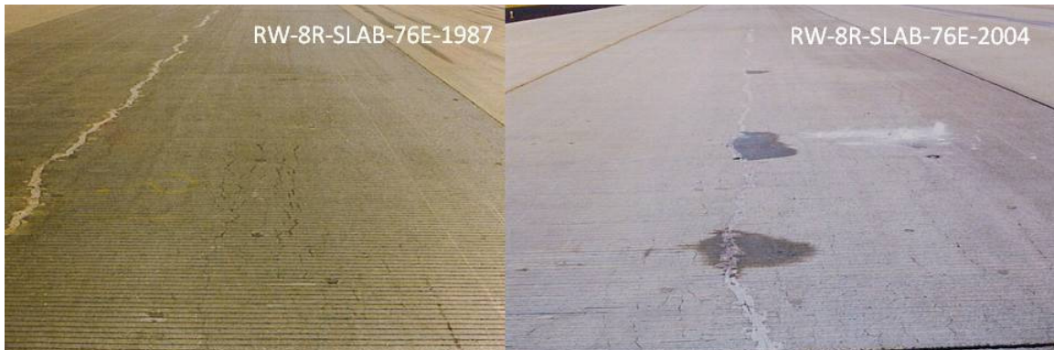
Figure 13 – Condition of Surface Cracking in RW-8R in 1987 and 2004
